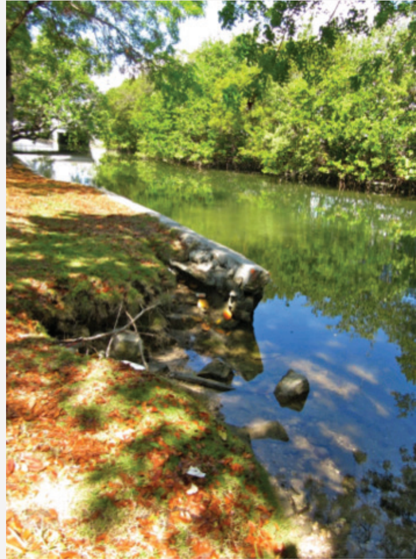
Figure 3. Eroded Portion of Canal Bulkhead (Source: City of Miami Beach)
