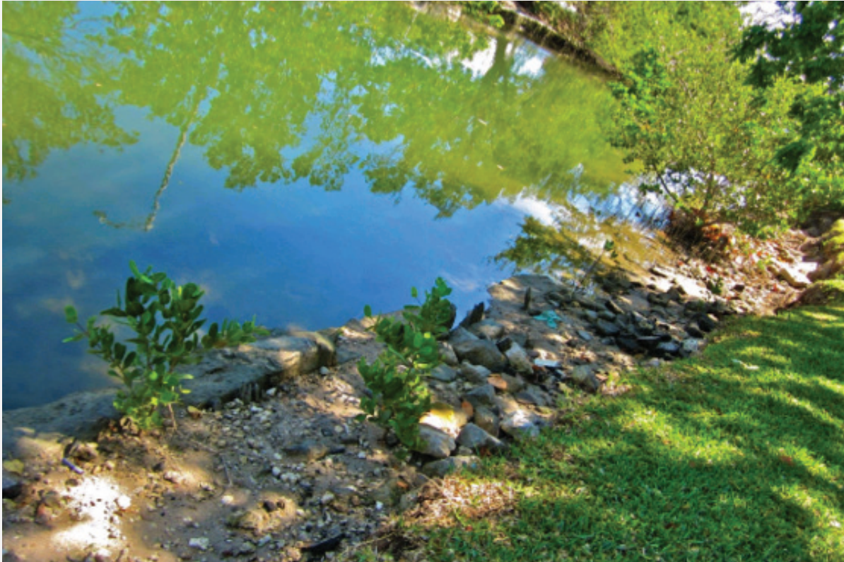
Figure 4. Erosion Behind Bulkhead (Source: City of Miami Beach)
